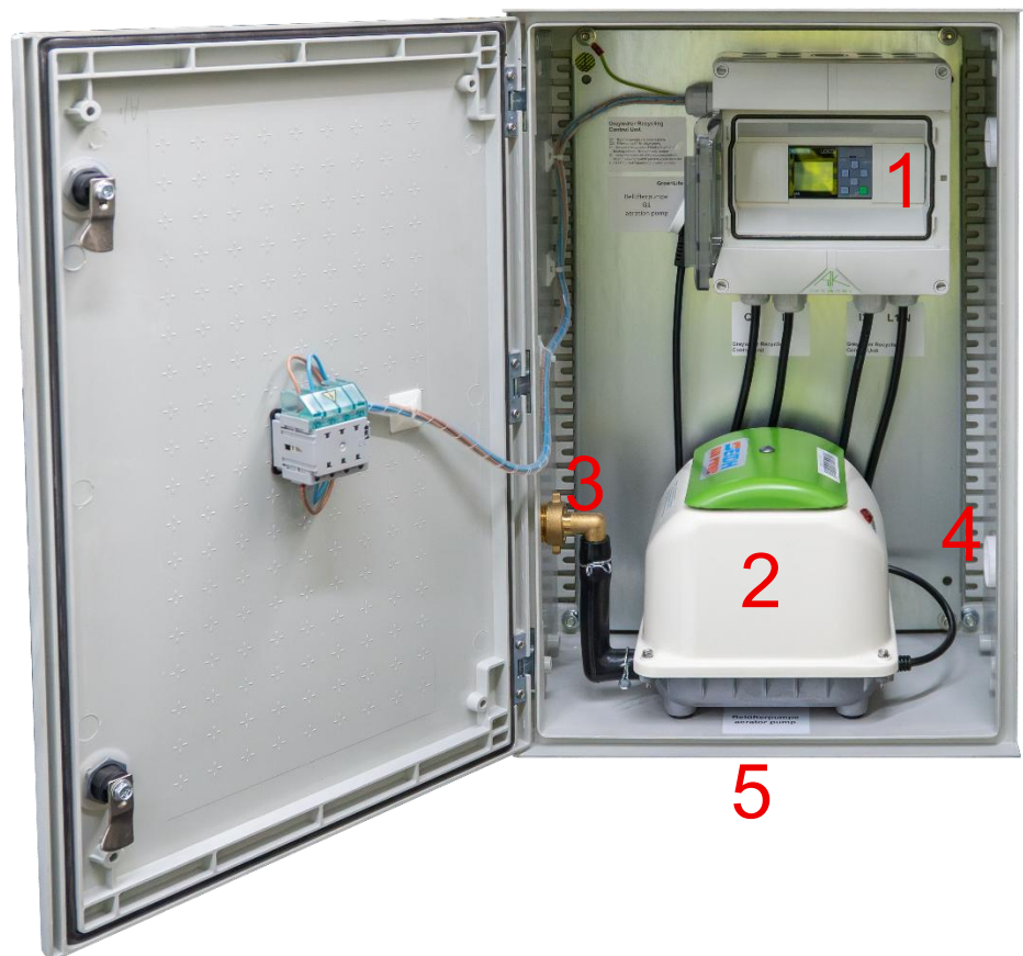
Figure 2: Control cabinet (variable)
